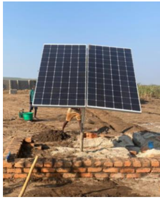
Solar panels to run pump.
